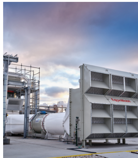
We recently completed the construction of a direct air capture (DAC) pilot plant in Baytown, Texas, to further develop a proprietary technology with the potential to significantly lower the cost of DAC.
